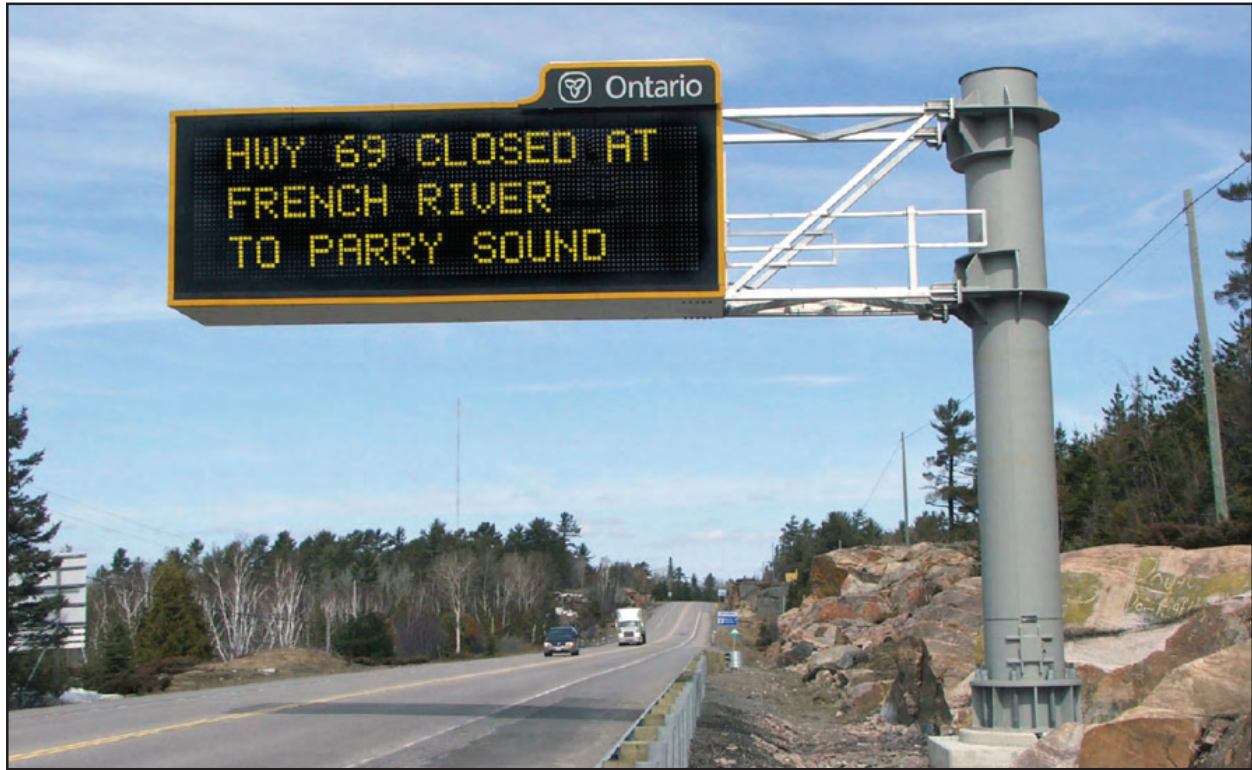
Figure 13 – MTO Roadside-Mounted (Cantilever) DMS
